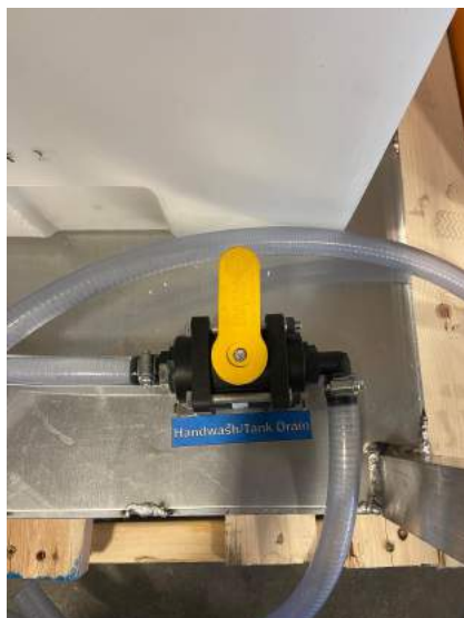
Drain Valve Closed *No water running*
