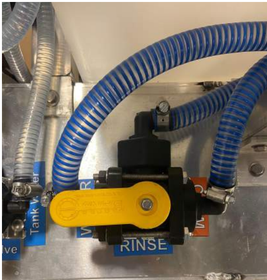
Chemical Line Valve Closed *Pulling from Water tank*
