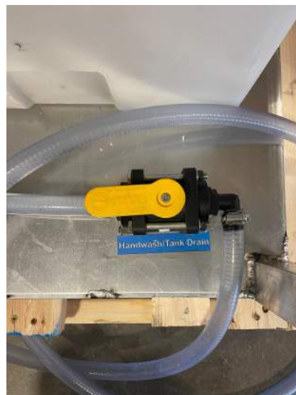
Drain Valve Open *Water running*
