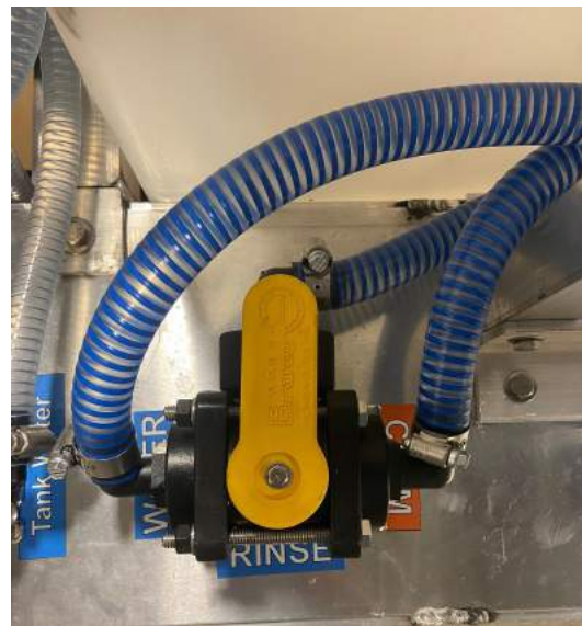
Chemical Line Valve Open *Pulling from Chemical tank*
